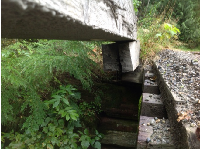
damaged riser block
